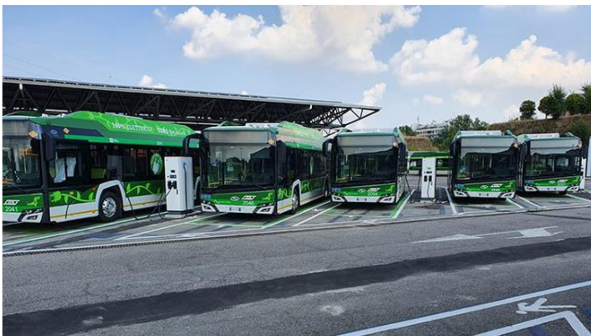
Photo 4: Electric Bus Charging Bay
