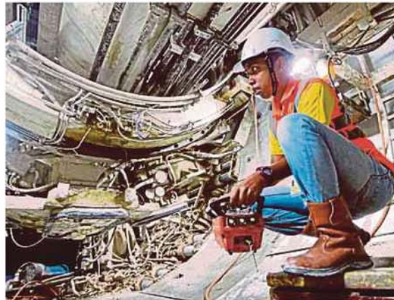
A worker at a Mass Rail Transit construction site in Kuala Lumpur last year. FILE PIC
