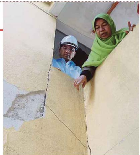
Housing and Local Government Minister Zuraida Kamaruddin inspecting the cracks that appeared at the Taman Keramat Permai flats in Ampang Jaya recently with Economic Affairs Minister Datuk Seri Azmin Ali. PIC BY MOHD YUSNI ARIFFIN
