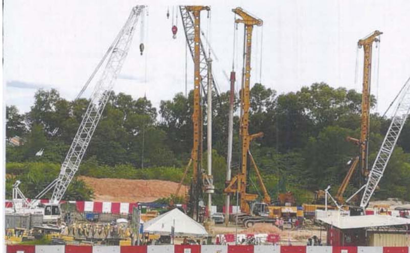
Drainage is an issue at construction sites as they have to make do with temporary drainage systems
